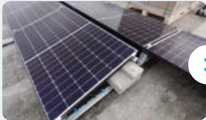
PV modules with ballast and mounting structure
