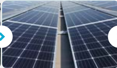
East-west arrangement of multiple string panels.
