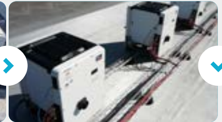
Three inverters placed on the roof
