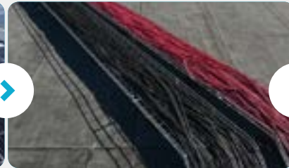
Cables from the different strings
