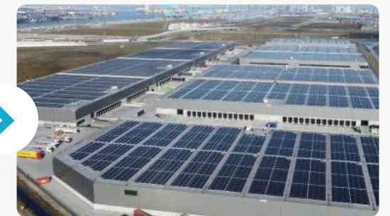
Completed rooftop installations (Maasvlakte ~2,5 MWp per roof)
