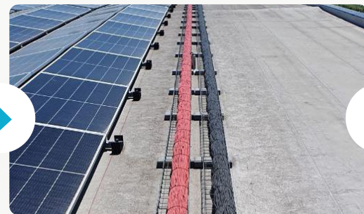
DC string cabling
