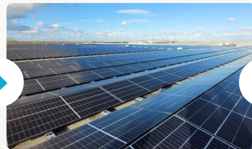
Panels_ east-west configuration
