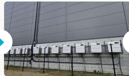
Inverters (installed on a facade)
