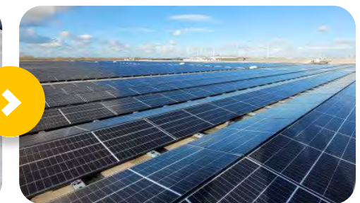
Panels in an east-west configuration
