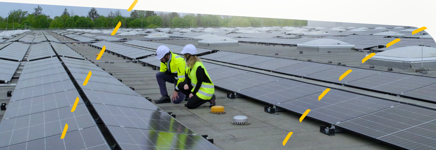
Sunrock's 5.2 MWp solar system powers Mercedes-Benz's Rastatt site with clean energy.
