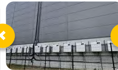
Inverters (installed on a facade)
